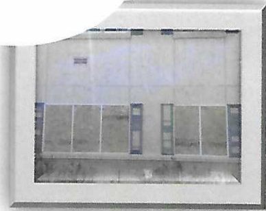
The EIFS, windows and shutters are left in shambles.
